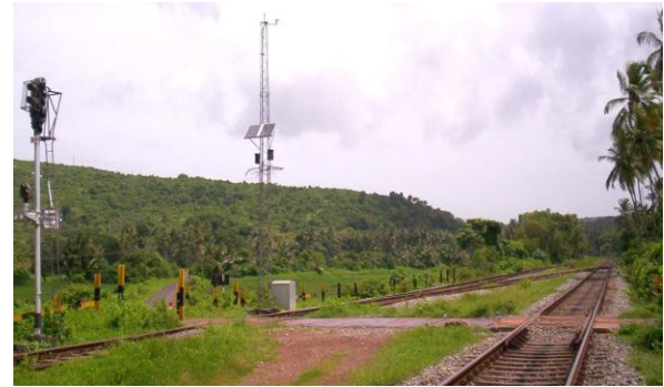
Fig 3: Showing a typical video based Gate System at an Un-Manned Level Crossing with ACD Accessories – Tower having the Hotter-Flasher Unit, Solar Power Panels (Close-up View) & the Location Box hosting the ACD Unit Legend:
