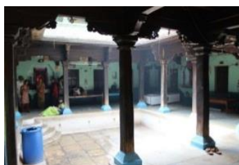
Fig8. Roof with A Wooden Column and A Metal Beam and Wooden Columns and Wooden Beams.
