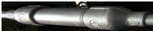
Fig. 2: Holding tube attached at hot milk outlet of shell and tube heat exchanger
