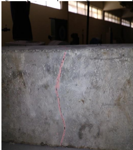
Fig. 3 crack pattern after loading of beam under point load
