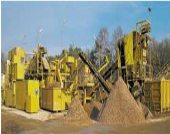
Aggregate crushing plant
