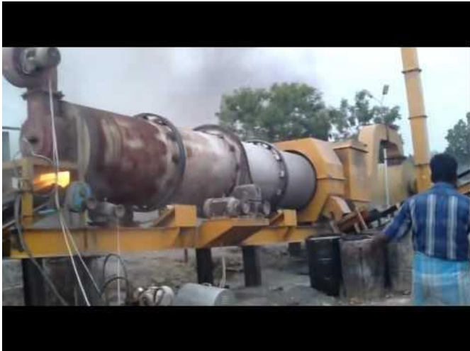
Fig. 9. Central mixing plant
