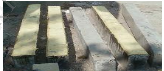
Figure.2 Application of epoxy - hardener and fixing of Kevlar fabric on the beam
