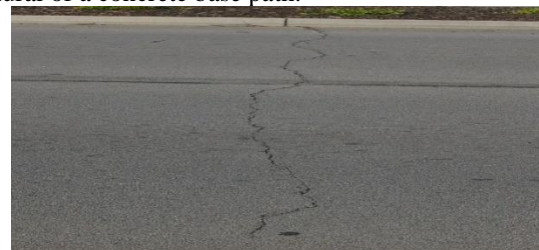
Figure: Transverse crack
