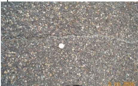
Figure: Low severity cracking
