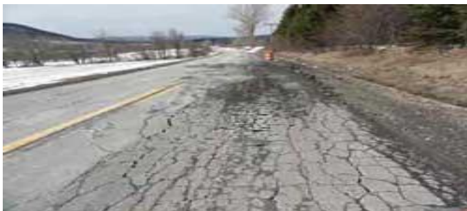
Figure: High Severity cracking
