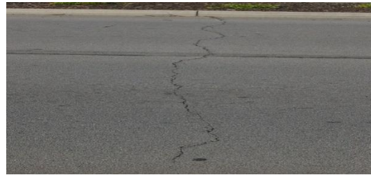
Figure: Transverse crack
