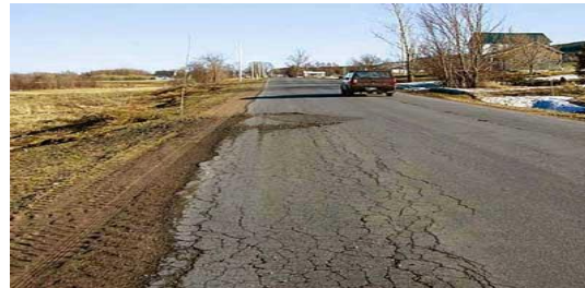
Figure: Edge cracking.
