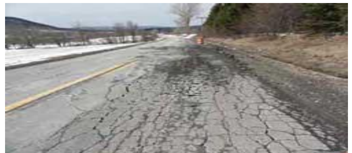
Figure: High Severity cracking
