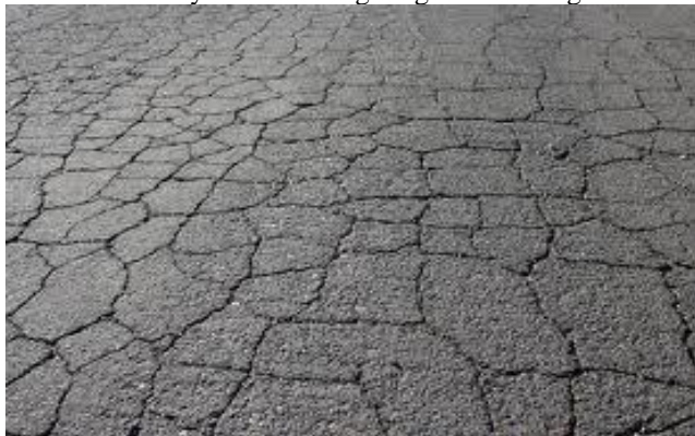
Figure: Alligator cracking.
