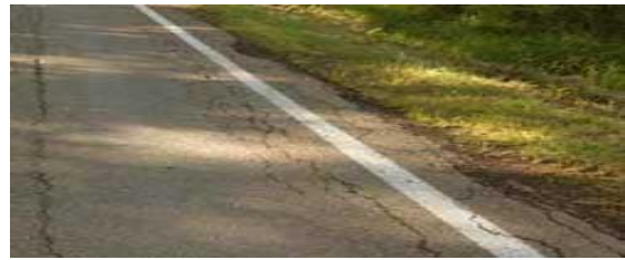
Figure: Medium severity cracking.
