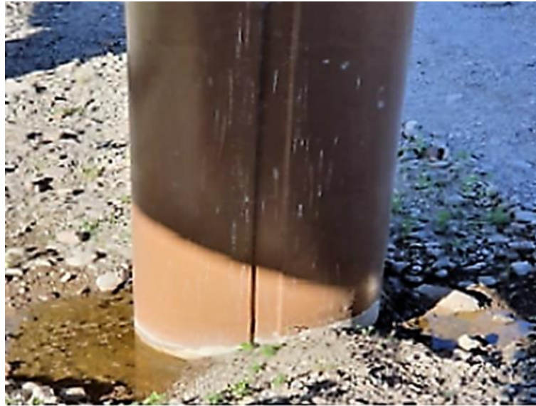
Fig. 2. Evidence of horseshoe vortex scour in bridge pier.
