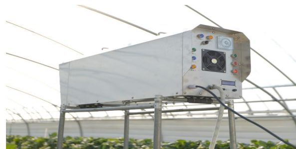
Fig. 2. The catalyst-type CO 2 generators.
