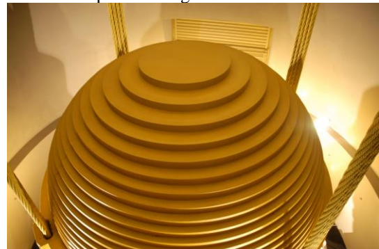
Fig 1: Tuned Mass Damper
