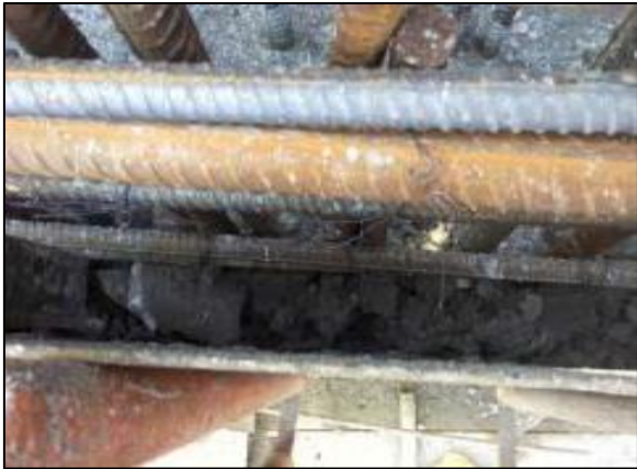
Fig-4: Lump formation problem in RCC chimney shell construction by Slip form technique.
