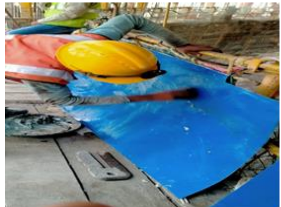
Fig-8: Making of sheet as per the size of plate used as a slip form shutter plate.
