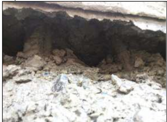
Fig-3: Concrete collapse problem in RCC chimney shell construction by Slip form technique.
