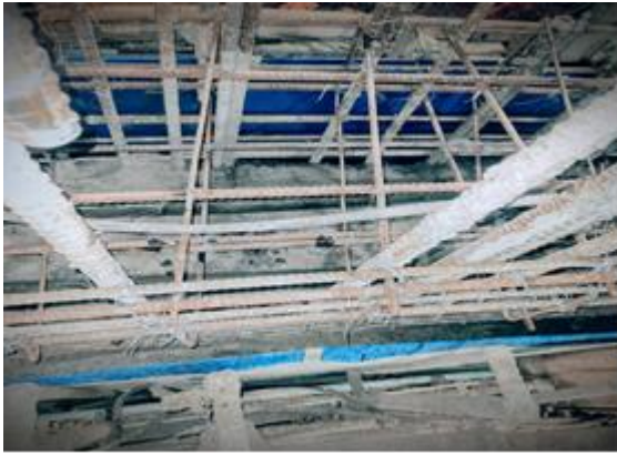
Fig-10: Fixing of sheet along with both inner & outer shutter plate considering the provision for making horizontal sliding.
