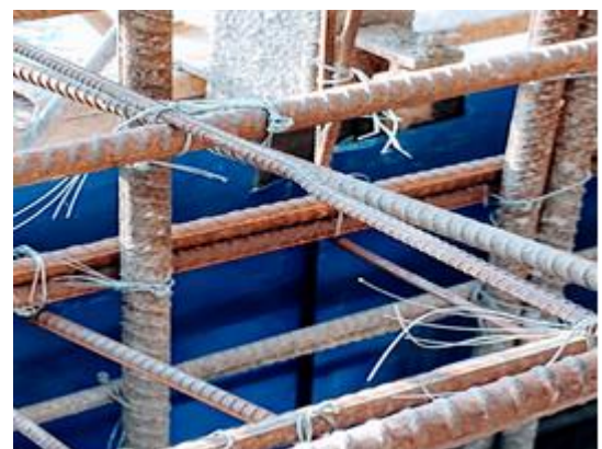
Fig-9: Fixing of sheet as per the size of plate used & considering the provision of slipping horizontally along with shutter plate.
