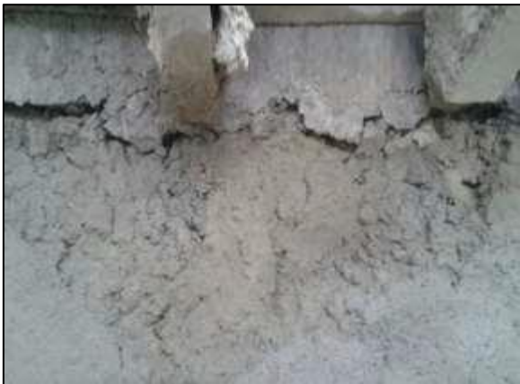
Fig-1: Lifting crack in RCC chimney shell construction by Slip form technique.
