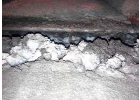
Fig-2: Delamination problem in RCC chimney shell construction by Slip form technique.
