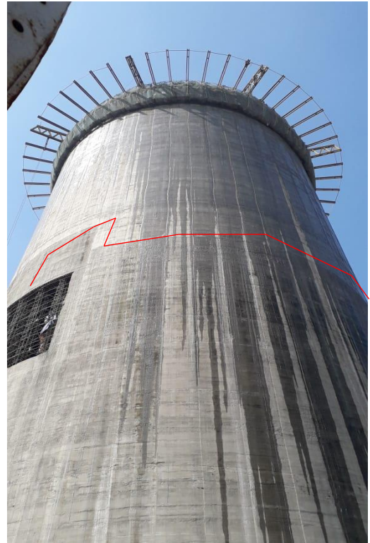
Fig-13: Concrete surface of RCC Chimney shell by using of 0.47 mm thick color coated galvanized sheet along with steel shutter plate for Upper part of chimney shell or without using of sheet Bottom part of shell.
