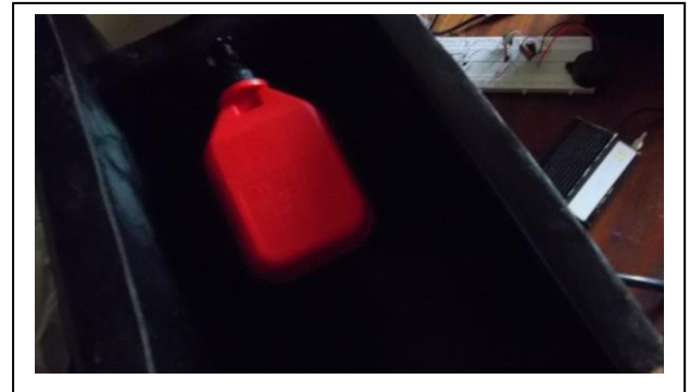
Fig. 3. Float switch inside a fabricated transformer compartment.
