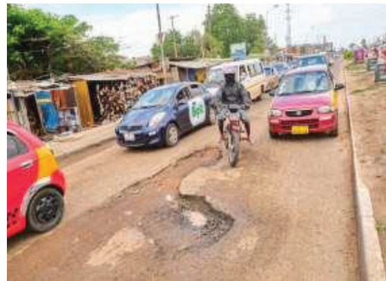
Fig. 4. Irregular, pothole-affected road conditions typical of West African urban networks.
