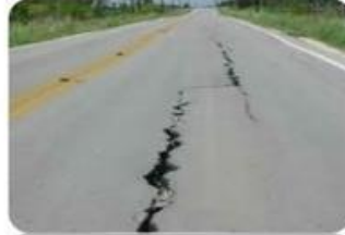
Longitudinal Cracks in Asphalt Flexible Pavement
