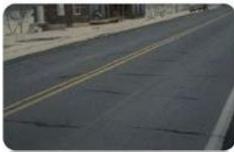
Transverse Cracking in Asphalt Flexible Pavement
