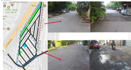
Figure 6. asphalt must be replaced with paving block Source: Author, 2017
