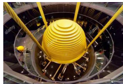
Fig.1 TMD installed in Taipei 101 tower
