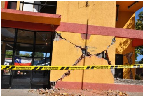
Fig. 4 - Shear wall failure during earthquakes
