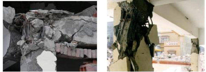
Fig. 2 - Columns failure during earthquakes
