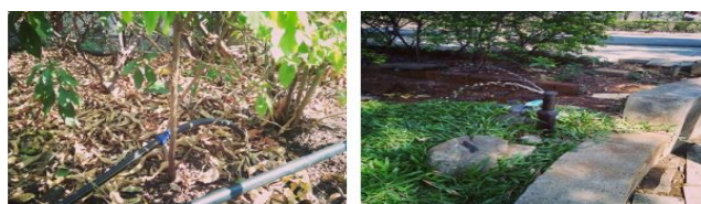
Fig.12 Water supply in the Garden area
