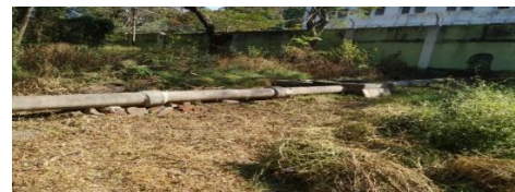
Fig. 11 Pipes Connected To the Treated Water Collection Tank
