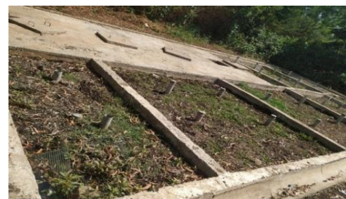
Fig.5 Bio Digester Tanks Attached To the Constructed Wetland Beds
