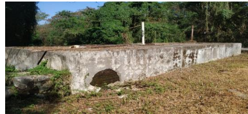
Fig. 10 Treated Water Collection Tank
