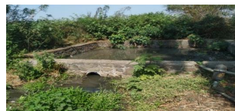
Fig. 6 Treated Water Collection Tank
