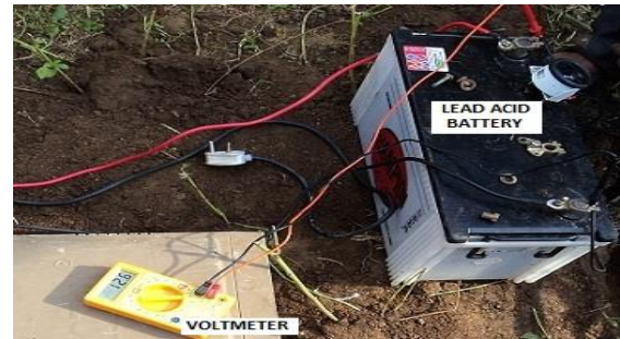
Figure 4: Lead acid battery and voltage testing by Voltmeter
