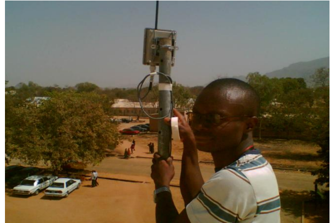
Fig 4.2 The 400mW Outdoor Access point/Bridge aligned to the digital centre.
