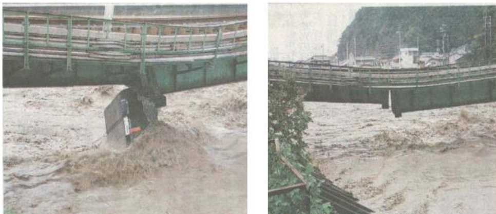
Figure 10. Loss of pier due to rotation of pier (Brioud et al. 2011)
