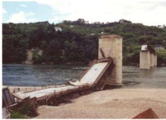
Figure 9. Loss of deck due to excess settlement of pier (Brioud et al. 2011)
