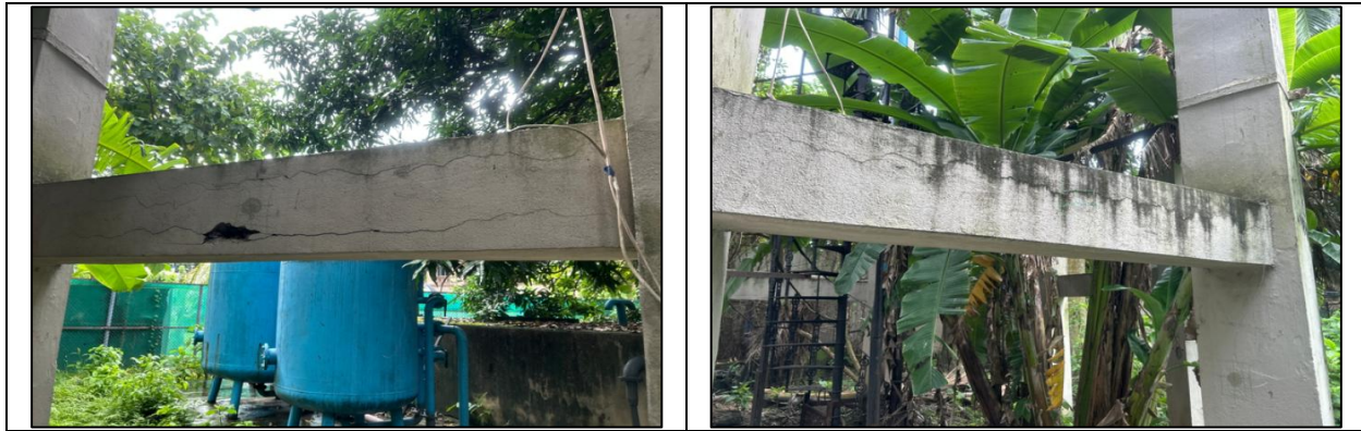
Photo 3, 4: Combination of Flexural & shear crack observed on beam.
