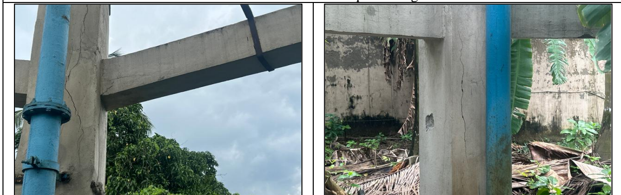
Photo 7, 8: Vertical cracks observed on column members.
