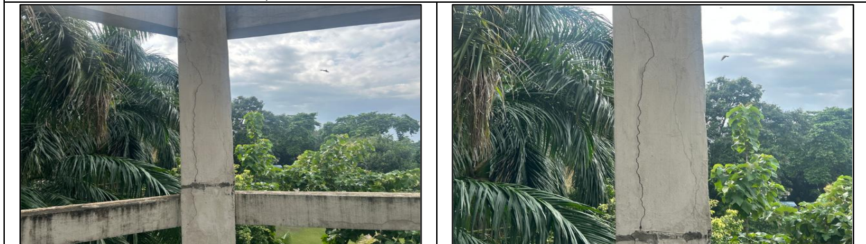
Photo 9, 10: Vertical cracks observed on column members.
