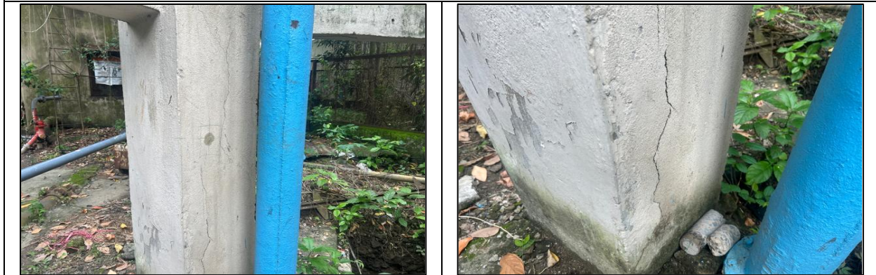
Photo 5, 6: Bulging of column with beginning of developing vertical cracks. The reason behind this is due to increase load/ inadequate design.
