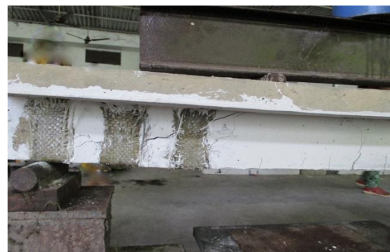
Fig 9 Debonding of GFRP strip followed by shear failure
