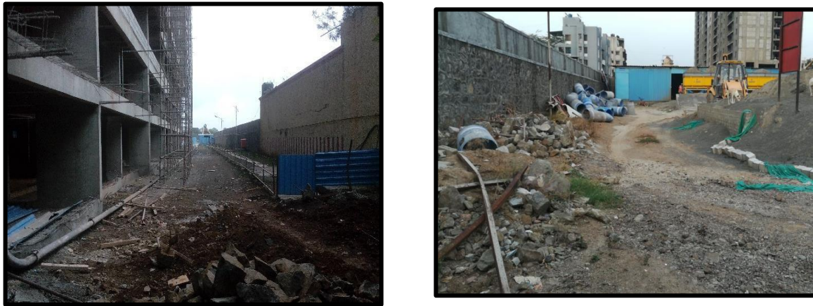
Fig 3.5: Stacking Of Formwork Material In Hazardous Manner On Site
