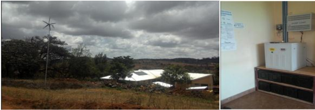
Figure 2: 1.5 kW Wind-Solar Hybrid System installed at Gidas Health Centre in Babati District Manyara Region
