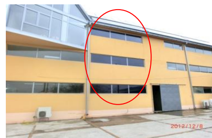
Figure 6. Installed window modules in the existing window frames of CS building. Left and right windows columns of the building are existing standard glasses; the middle column of windows (circled in red) are CS-modules.
