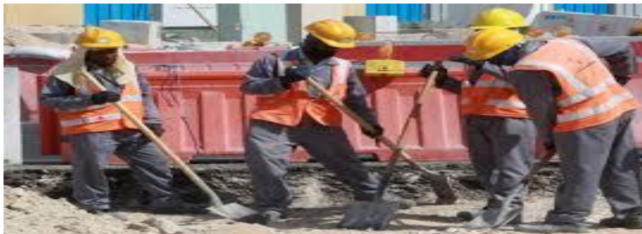
Figure: Picture showing workers working with safety equipments, which are helmet and gloves.
