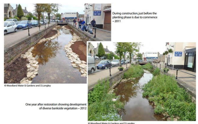
Figure 4 Pictures of berm creation during construction and one year after showing vegetation colonization on the River Somer in Midsomer Norton in Somerset
