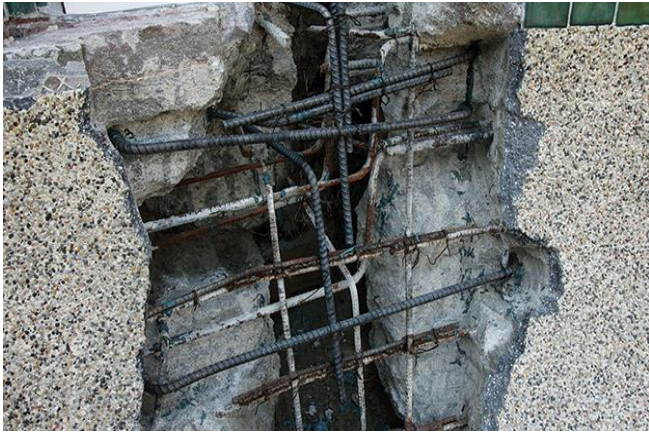
Fig. Damaged structure
