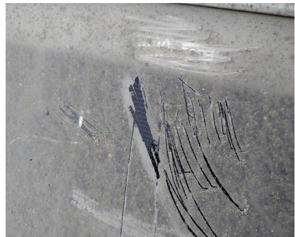
Fig. 2. Hardened cement on solar panel
