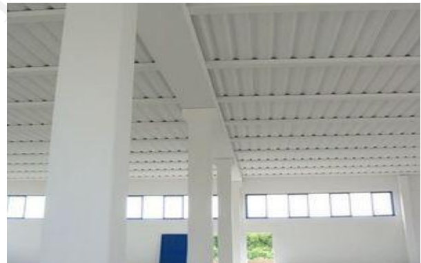
Figure 5. Wide Beam for a meeting hall
