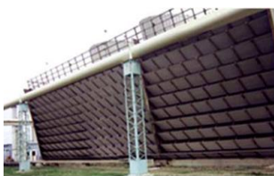
Figure-4 Timber made Cooling Tower
