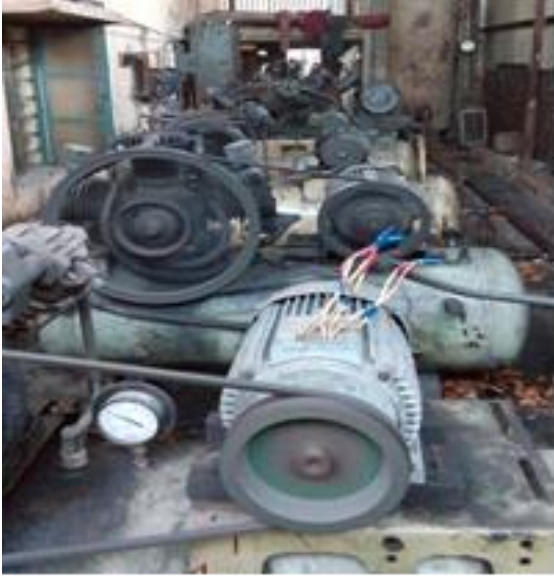
Fig. 3. Air Compressor with air receiver
