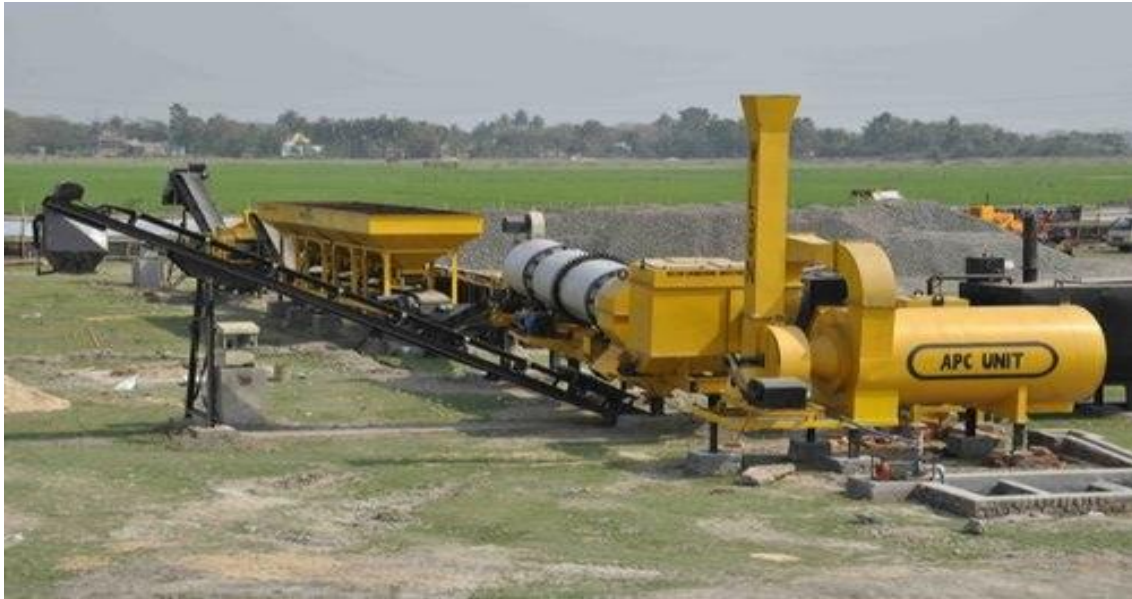
Fig 9: Central mixing plant
