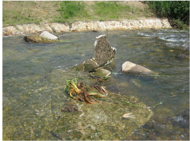
Pieces of collapsed pillars & ripped off the concrete slab of the stilling basin. February 2012. (Photo: Mumba Kolala).
