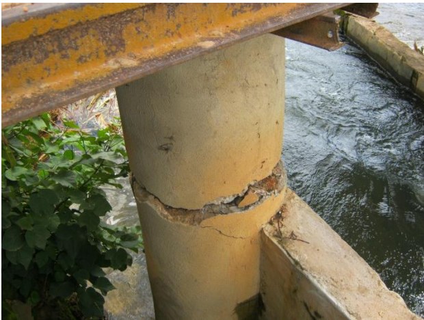
One of the two (2) severely fractured pillars that were left standing. February 2012. (Photo: Mumba Kolala).
