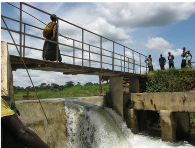
Fig 1b; Traces of debris left behind hanging on one of the pillars of St Marys dam in the aftermath of the attempted dam failure. Note that only two (but fractured) pillars were left standing. February 2012. (Photo: Mumba Kolala).
