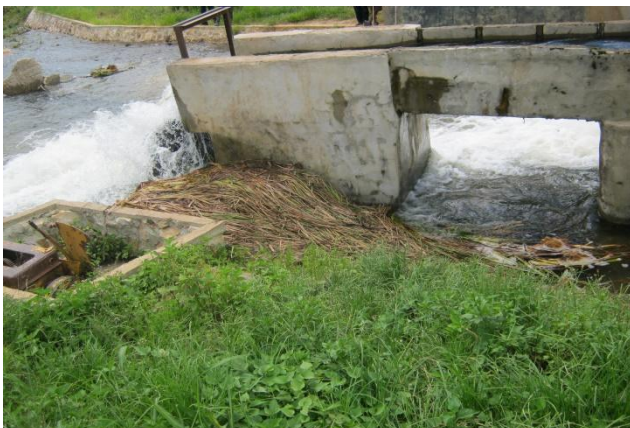
Stilling basin with deposited debris of some of the masses of Typha Plants that bypassed the spillway after the attempted failure February 2012 (Photo: Mumba Kolala).
