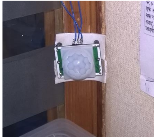
Fig.4. PIR sensor installed at a cubicle
