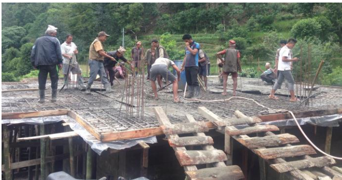
Compressed Earth Block and RCC roof structure of a new house post earthquake.
