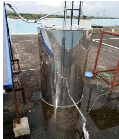
Fig.2 Thermal storage tank
