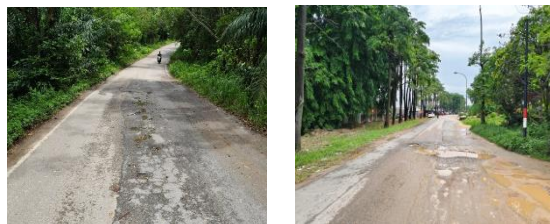
Figure 1.1 Condition of road
