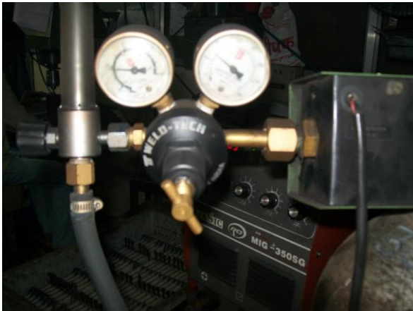
Figure 4 Gas Preheater and Pressure Regulator
