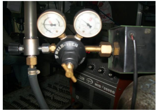
Figure 4 Gas Preheater and Pressure Regulator
