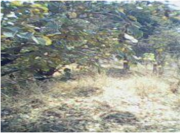
Figure 14; Guyaku Dam2 Poorly Maintained Embankment
