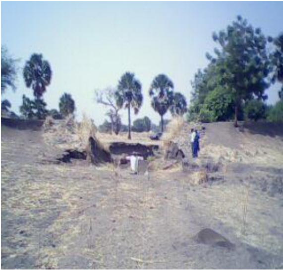
Figure 2; Spillway Failure at Nzuzu Dam Garkida
