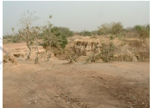
Figure 5; Water overtops and cuts the dam forming a gully
