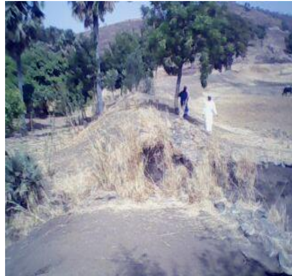
Figure 3; Failure as viewed from Dam crest
