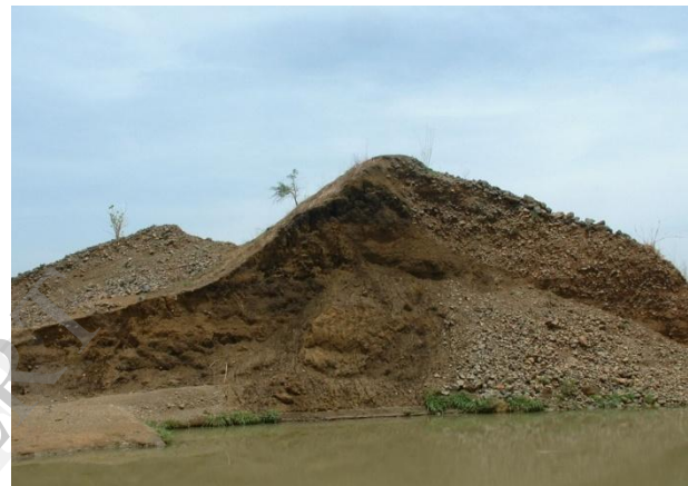
Figure 17; Crossection through the Embankment of Cham Dam in Gombe at the point of failure
