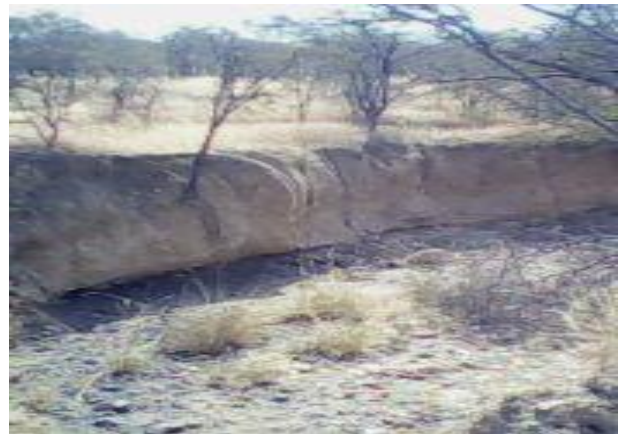
Figure 15; A Gully cut the Embankment at the right Abutment
