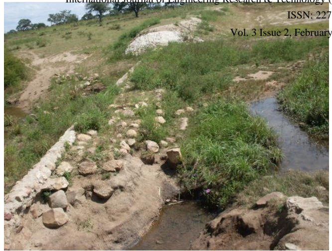
Figure 9; Dull Dam Spilway Failure in Tafawabalewa Bauchi
