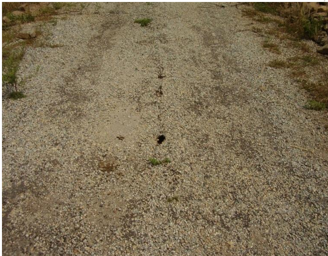
Figure 12; Cracks on the embankment crest at Waya Dam Bauchi
