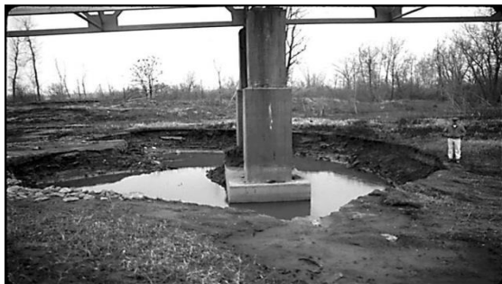
Fig.2: a picture showing the local scour around a bridge pier
