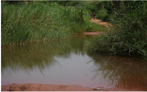
Plate 6B: Other side of damaged Culvert on Stream Sumampa o the Owuo Buohoo road.
