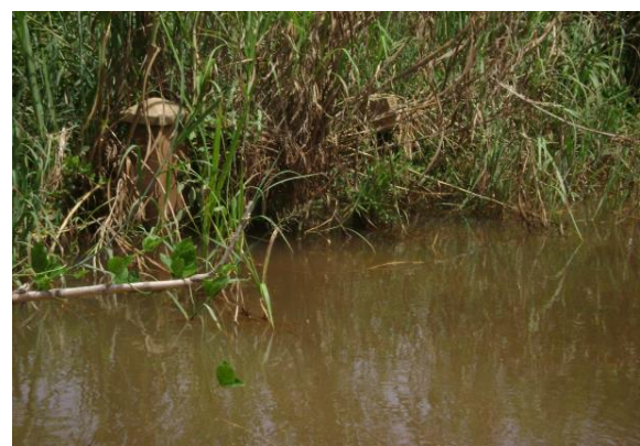
Plate 6A: One side of damaged culvert on Stream Sumampa on the Owuo Buohoo road.
