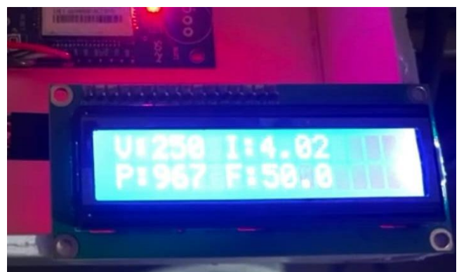
Fig.8 The LCD display showing real-time reading of the electrical parameters when a load is connected, and its range is above the threshold limits.
