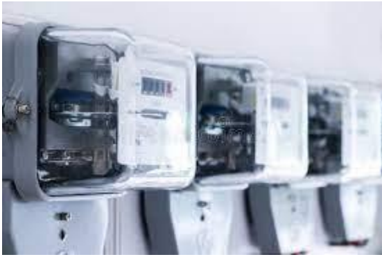
Fig. 5: Digital Energy Meters
