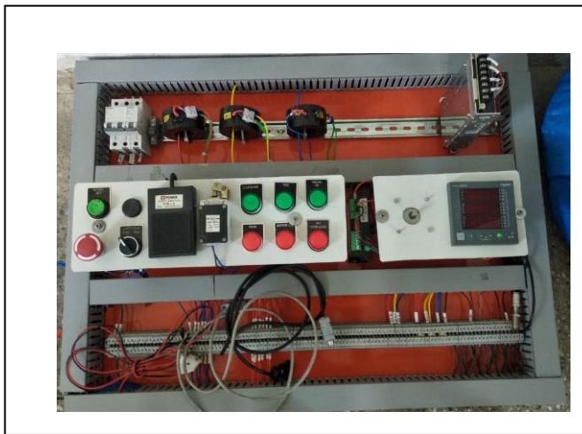
Fig. 4. Panel Assembly for Input-Output Connection.
