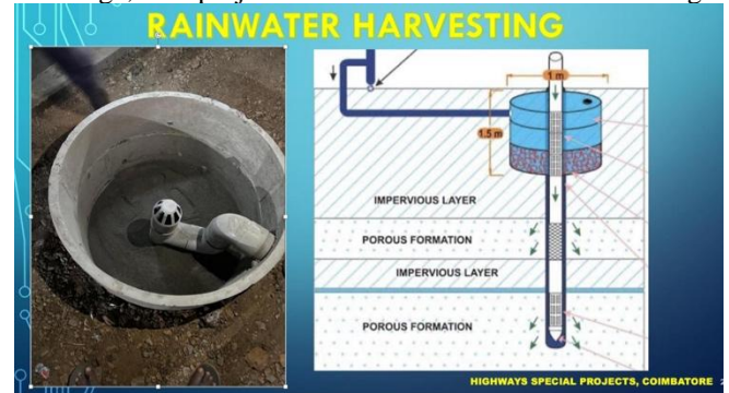
Fig 42. Rain Water Harvesting System
