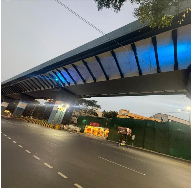
Fig 48. RGB Lighting at deck bottom in Junctions.
