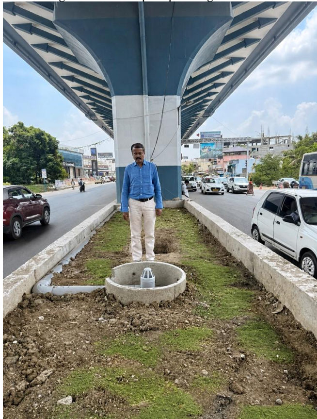
Fig 43. Drainage Pipe Connected to RWH System
