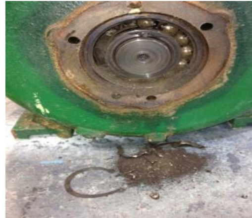
Figure 1: Rusting due to low life grease in bearing
